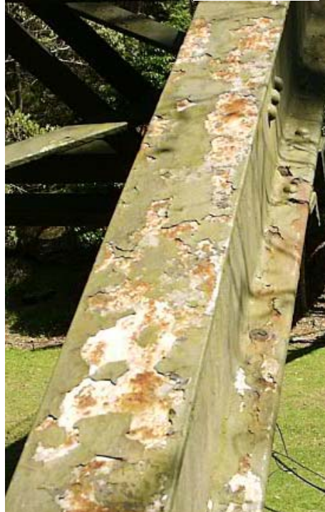
Reid Park Aqueduct – Coating assessment and repair specification
